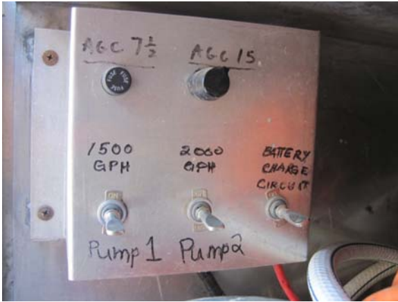
Picture G: Pump switch/fuses
