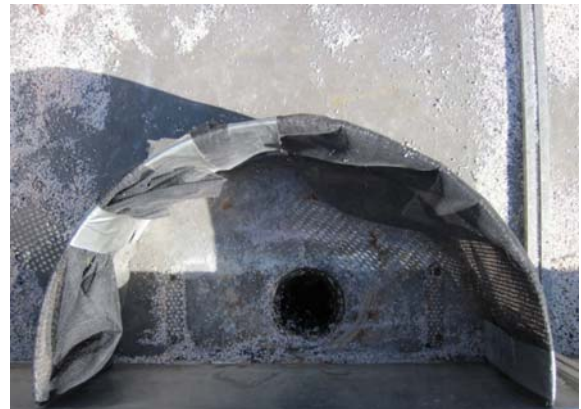
Picture J: Grit filter and screen
