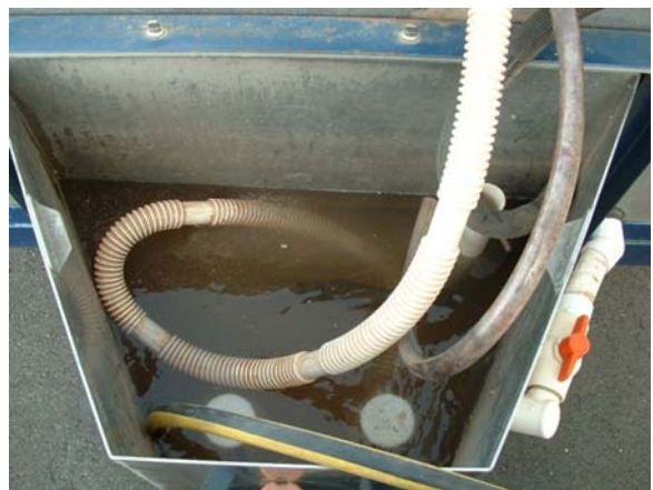
Picture F: Pump Compartment
