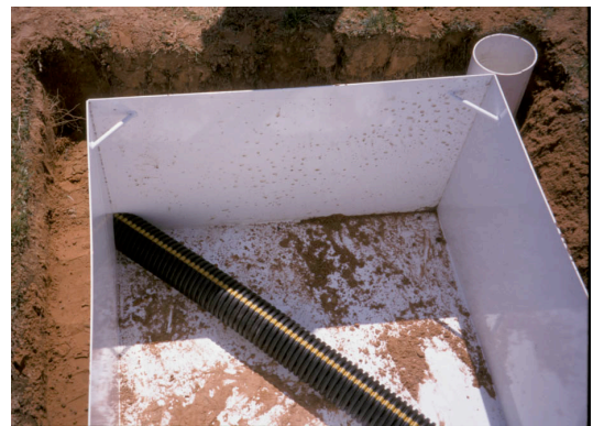
FIGURE 3. PLASTIC PERFORATED DRAIN PIPE IN LYSIMETER BOTTOM AND CORNER RAIN GAGE WELL (SOUTHGATE, APR 2004)
