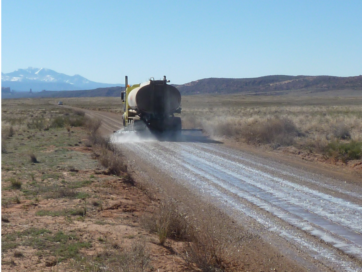
Figure 11. Application of MgCl_2 to the Salt Valley Road in Arches National Park.
