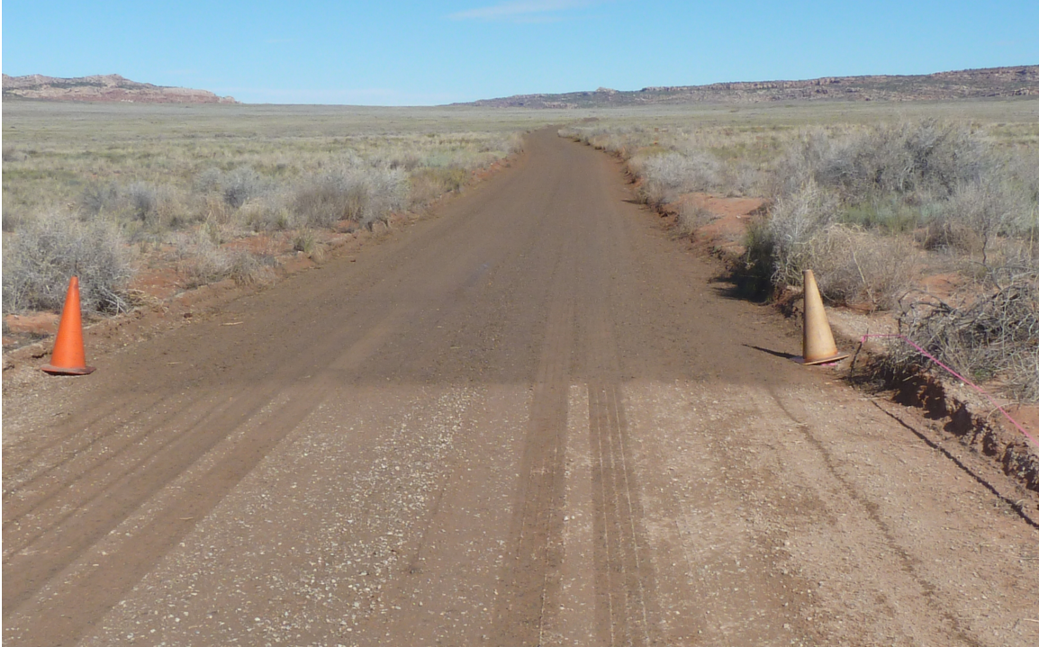
Figure 12. Following treatment with MgCl_2 a road will maintain a moist appearance as the MgCl_2 compaction layer at the surface continues to absorb H_2O from the atmosphere, thus inhibiting dust emission.
