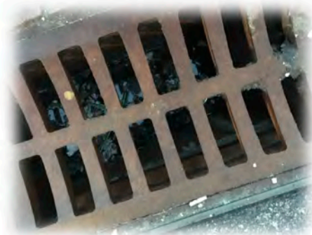
Catchment cover (grate)
