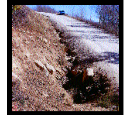
When ditches are used with insloped roads, drain runoff through culverts or into adjacent vegetation to filter sediment.
