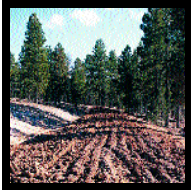
Roads may need to be ripped before they are closed. This will allow vegetation to grow more easily on the abandoned road.
