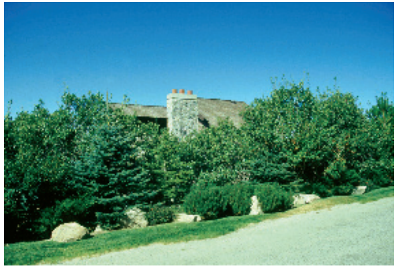
Continuous fuels and a wood roof increase this home's risk for damage from a wildfire.
