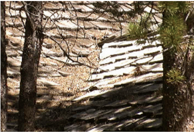
This home has a triple threat: wood shake roof, pine trees overhanging the house, and dead needles and other debris collected on the roof.
