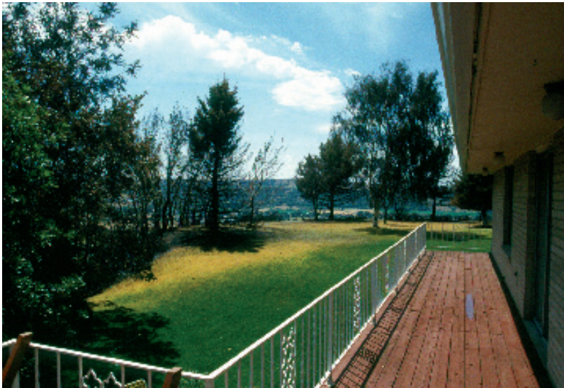
This home’s green, moist vegetation and setback from the hillside prevented it from igniting in the fire that burned up the hill. The wooden deck is a problem, and should be replaced with non-flammable material.
