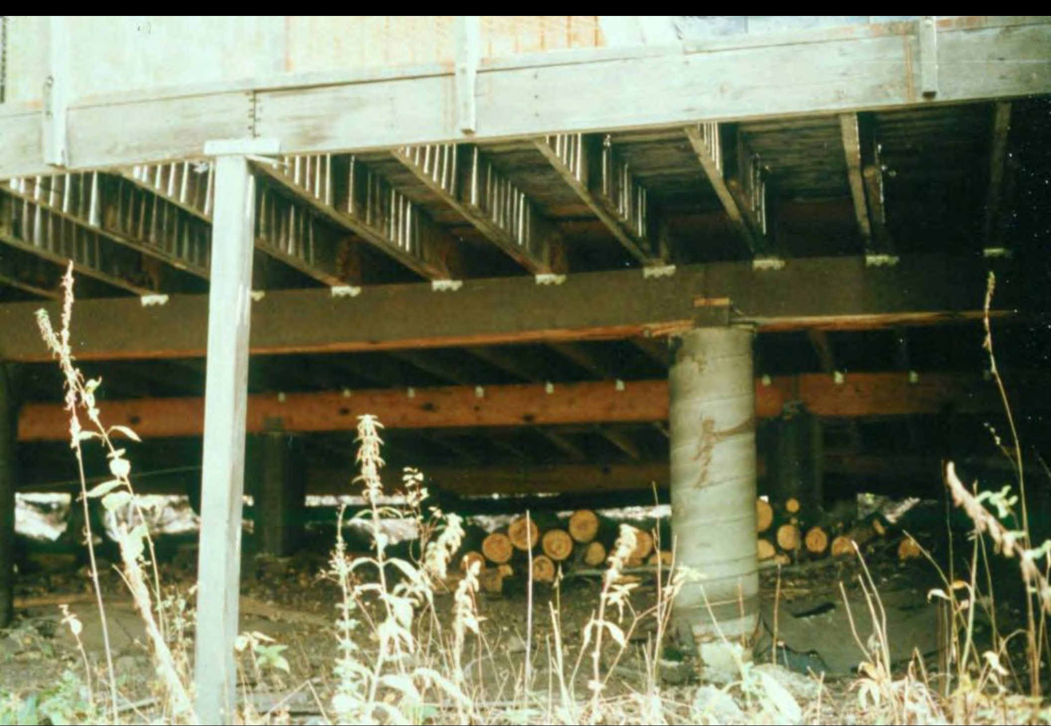
Firewood under wood deck
