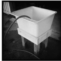
What is wrong with this picture?
