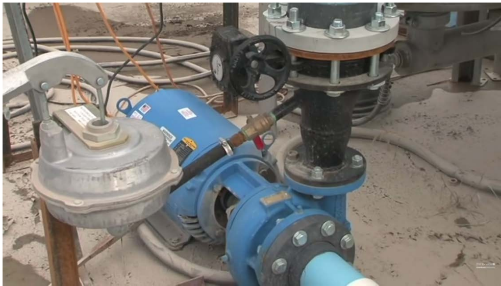
Figure 2. Pump for commercial drip irrigation system.
