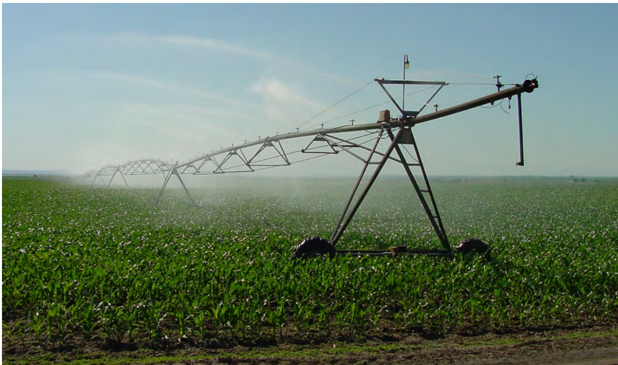
Figure 34. A center pivot with high pressure impact sprinklers on the top of the pipe. Around 40% of the water that leaves the nozzles cannot be collected in catch cans at the soil surface.
