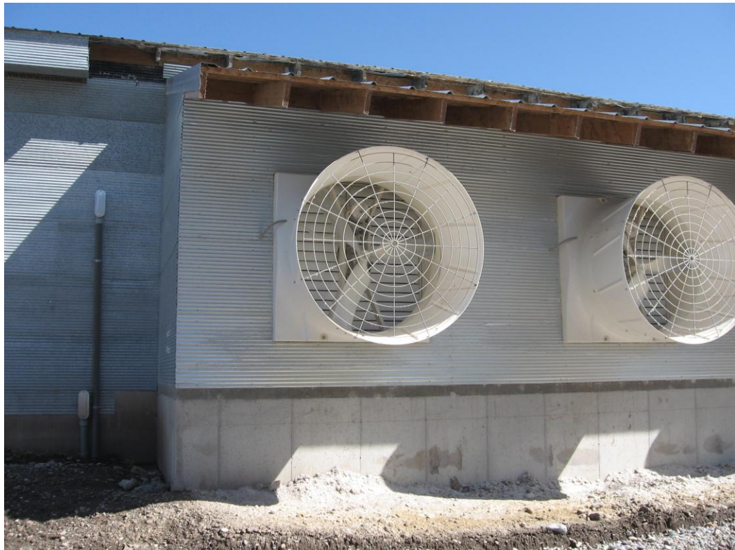
Figure 1. Fan installed on a poultry barn showing the discharge cones, louvers and protective metal nets.
