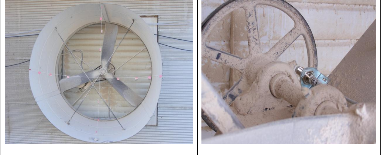
Figure 5. Location of induction sensor of fan motor
