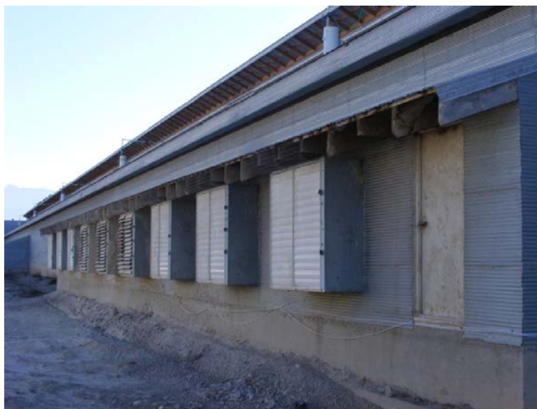
Figure 3. Manure-belt building (Building 4) external exhaust fans.
