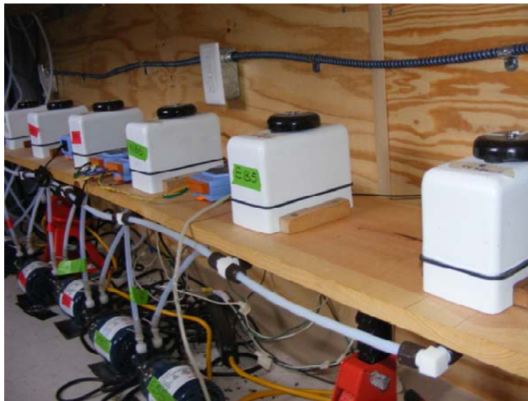
Figure 9. Custom-built gas sampling valving system.
