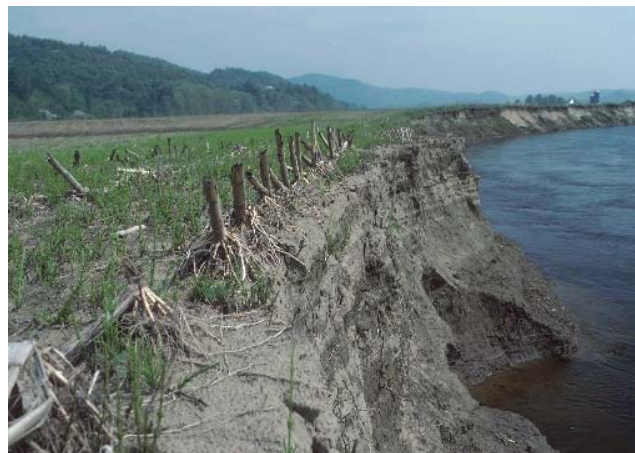
Eroding stream bank (Photo by USDA NRCS)
