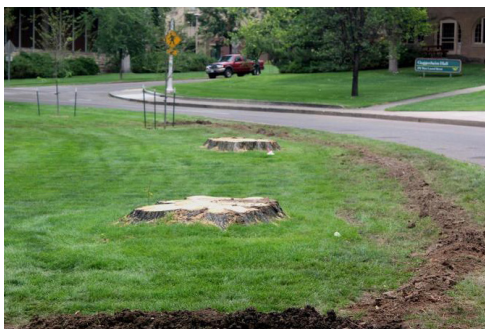
Trenching around newly removed elms to prevent root graft transmission of Dutch elm disease. Whitney Cranshaw, Colorado State University, Bugwood.org
