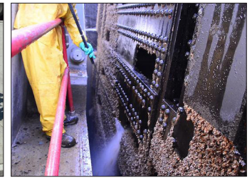
Fig. 12. Routine cleaning of quagga mussels from penstock gates at Glen Canyon Power Plant.
