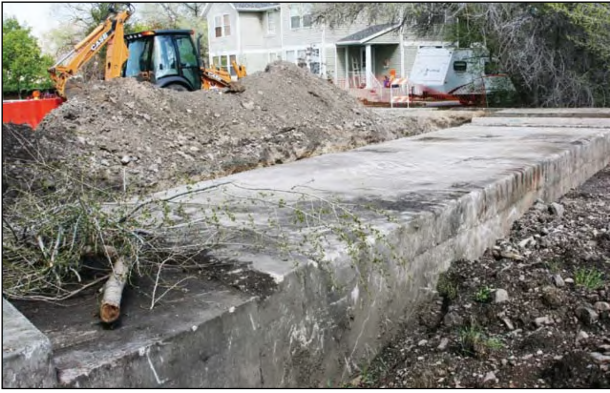
BRIGHAM CITY CREWS are in the process of repairing the bridge over Box Elder Creek located at 400 North. The bridge has been closed for months after a survey of bridges revealed damage, wear and tear on the structure.
